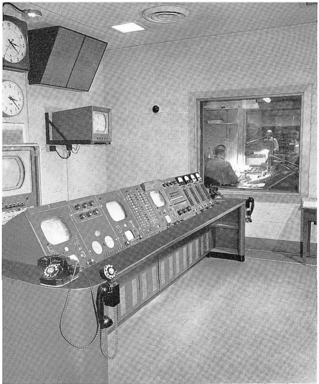
FIG. 22. Master Control facilities at this console include audio and video switching panels, master monitors and an audio ringdown and remote panel. The booth shown is the Studio "X" announce booth where any or all of the four outgoing audio channels can be overridden.
